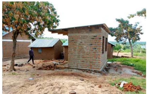
Roofing, plastering and pointing of brickwork joints of temporary kitchen in Emmanuel Primary School
